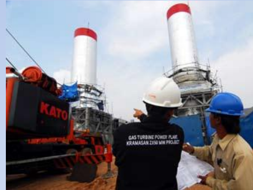
2 x 57 MW PLTG/ GTPP Keramasan, Sumatera Selatan/South Sumatera
